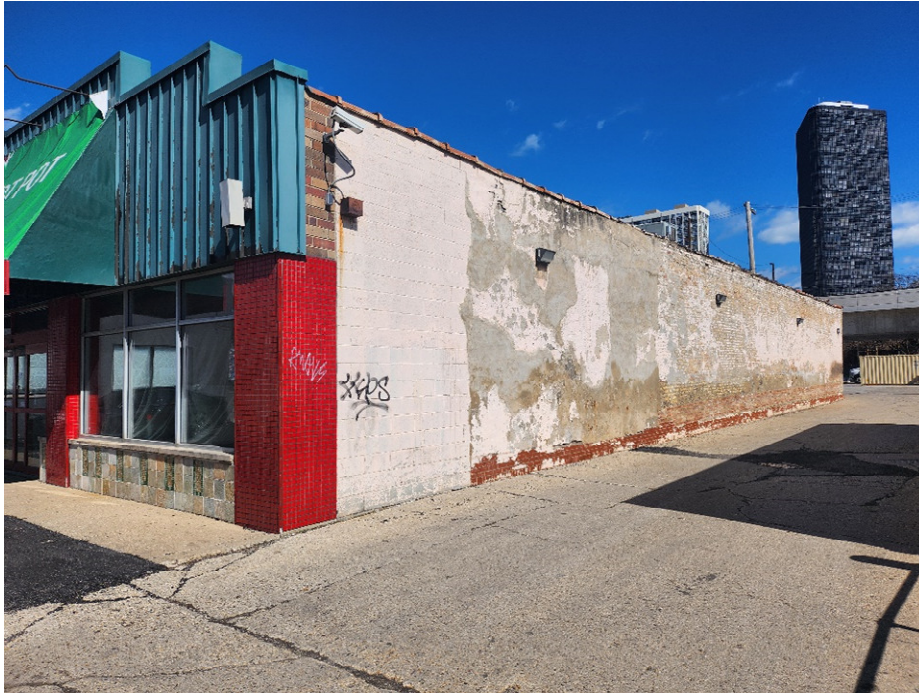
Exhibit 1: South facing wall at 5353 N. Broadway
